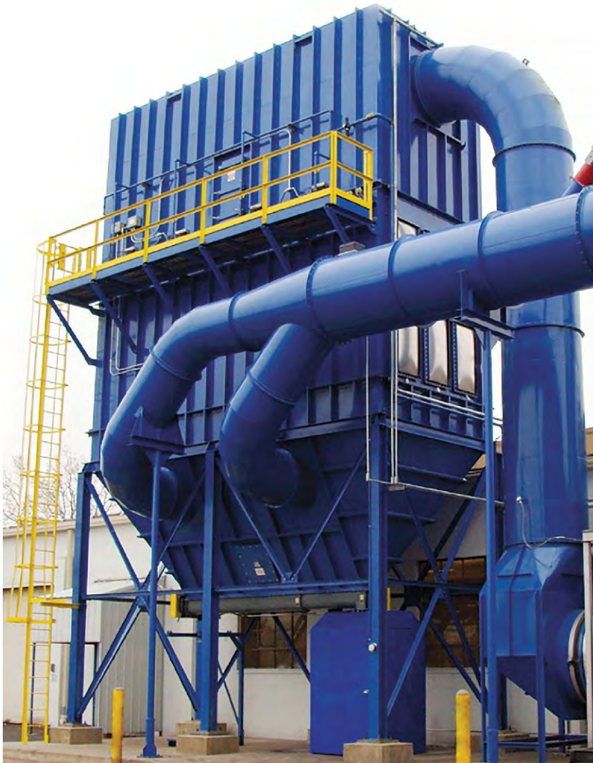
Schust fabricated and installed new 12-gauge mild steel ductwork from the existing wet scrubber to a new fan inlet.
