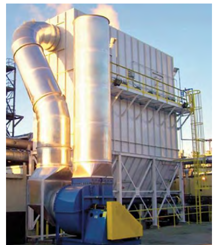
The single dust collector module system for the facility's sand system has been able to accommodate the business's expansion.
